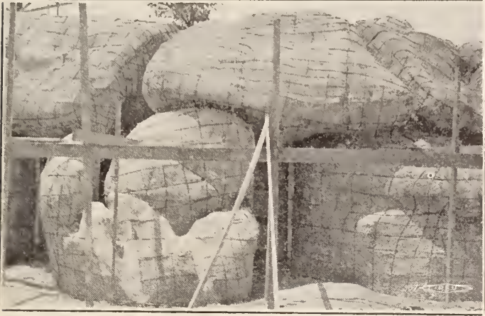
3. A close-up showing boulders lathed and scratch coated inside. Ready to receive second or heavy coat.
